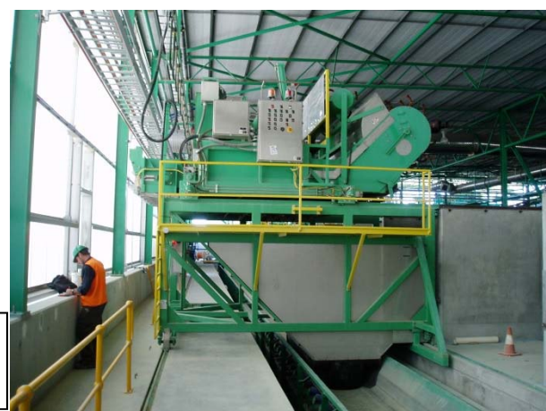
Automated Bay Unloading
