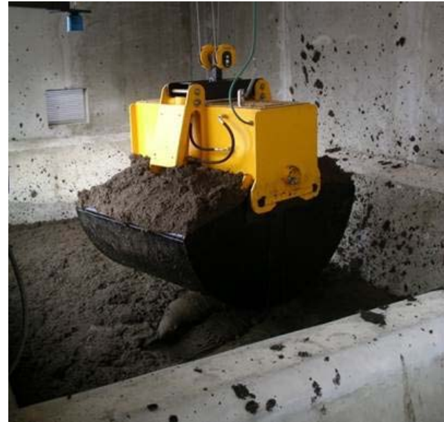
Biosolids Storage Bin
