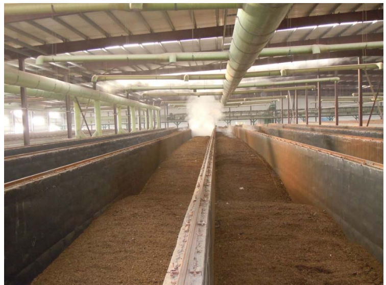
Agitator Working in Bay Under "Targeted" Ventilation Duct
