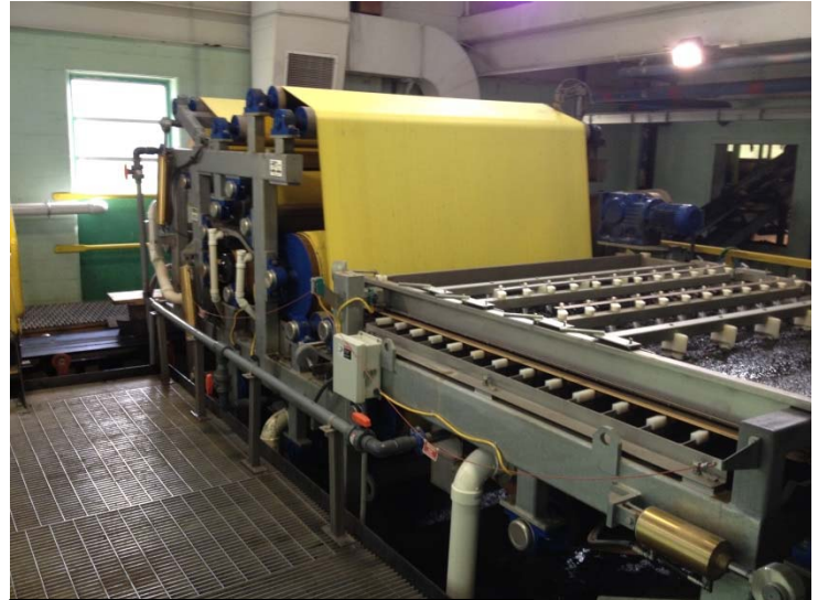
BDP Belt Press in Lockport WWTP
